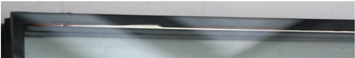
Figure 4 Insufficient butyl covering on a spacer
